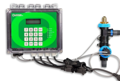
Cooling Tower Controller
